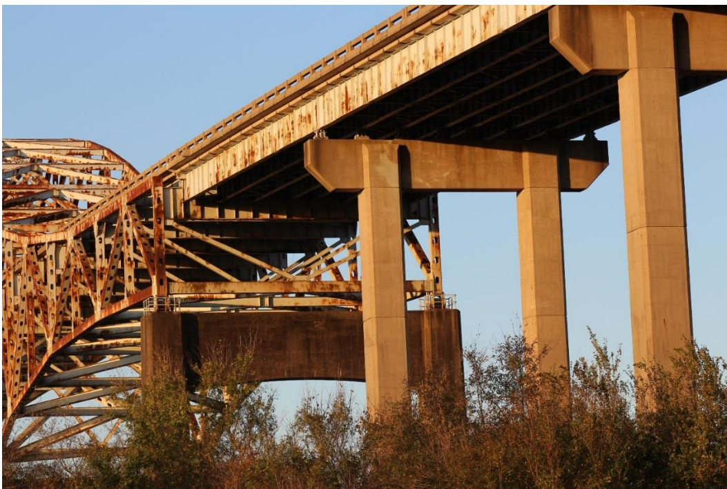
Condition Photo 4: Steel plate girders paint failure.
