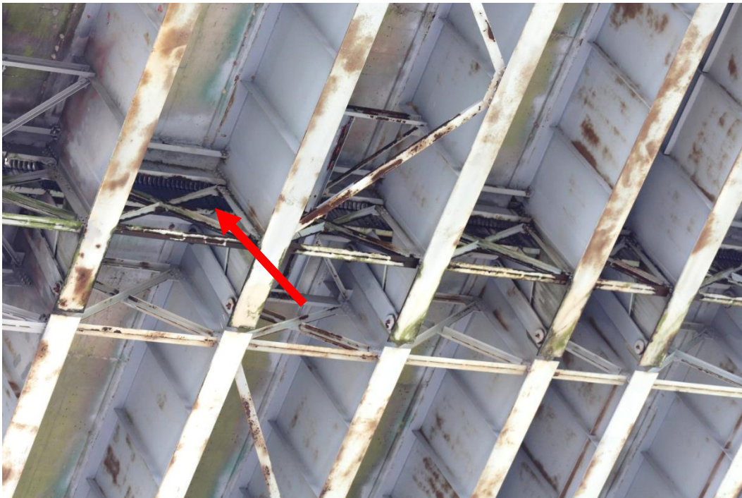
Condition Photo 8: Condition of steel plate girders hinged expansion joints, and condition of cross frames under the deck joints. Cross frames connection plates (hard to see in photo) also have paint failure, corrosion, and minor section loss, typical at cross frames under expansion joints.
