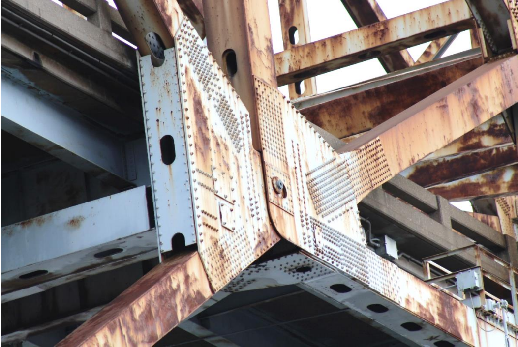
Condition Photo 5: Condition of hinged pin joint at truss span panel point L9; joint apparently frozen in full contraction position.
