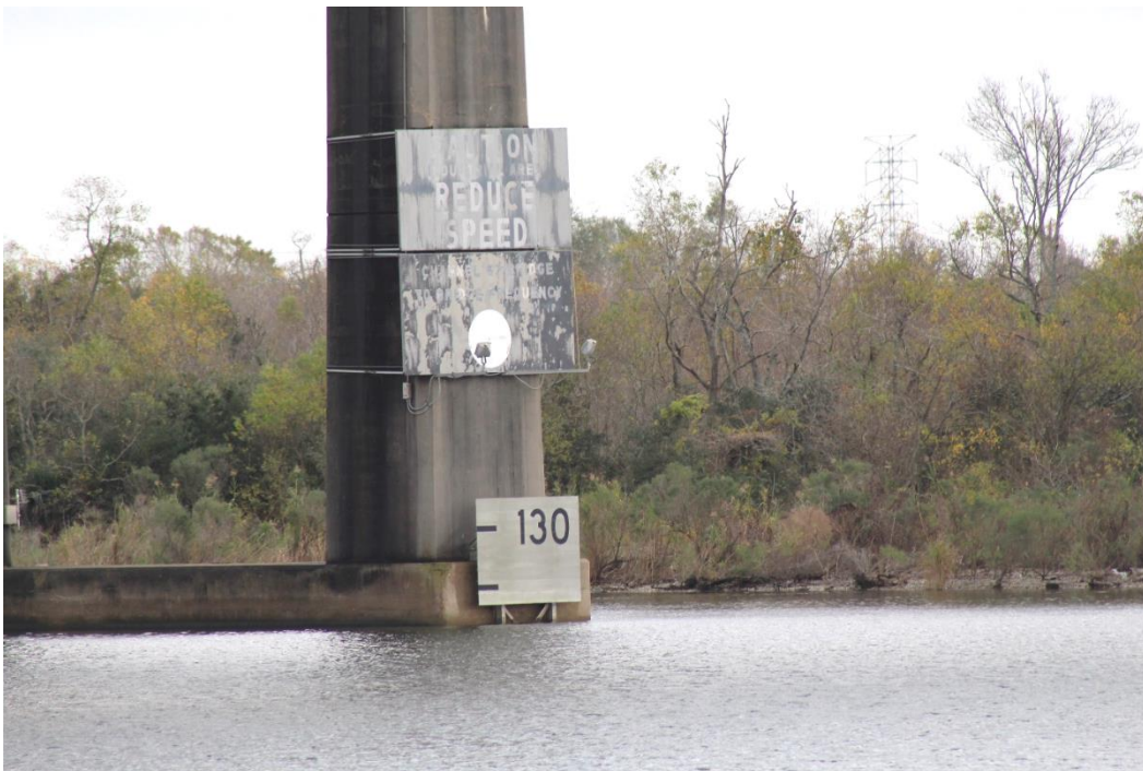
Condition Photo 12: Condition of waterway marking signs on pier in waterway, typical for two piers. Signs could be re-painted for easier reading.
