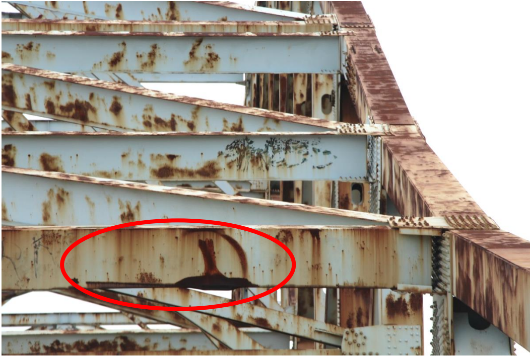
Condition Photo 9: Minor impact damage to end of portal member on the north end of bridge, over outside southbound traffic lane (horizontal member in foreground with dark rust and paint failure).
