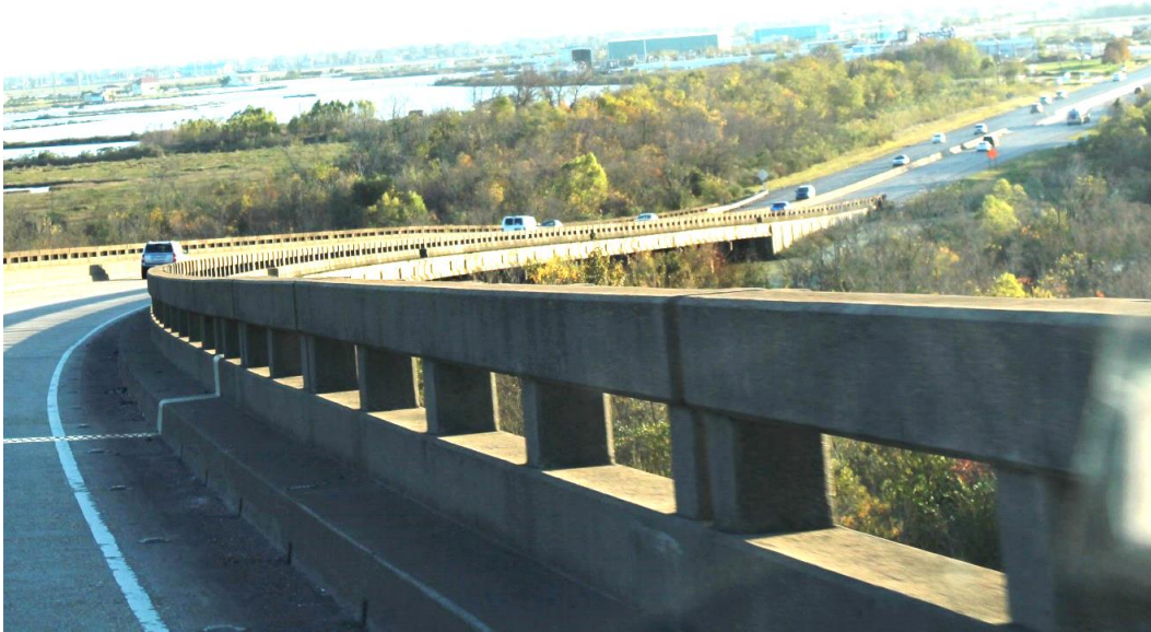
Condition Photo 3: Substandard concrete post and beam bridge railing, typical on entire bridge except at north end, west side, and where newer ramp was added with concrete Jersey-type parapet.
