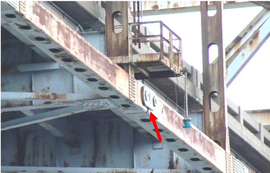
Condition Photo 6: Condition of hinged pin joint at truss span panel point L16.
