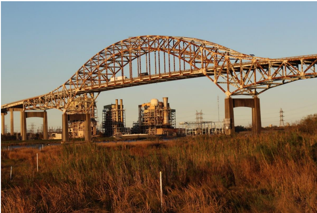
Condition Photo 2: Truss span paint failure.
