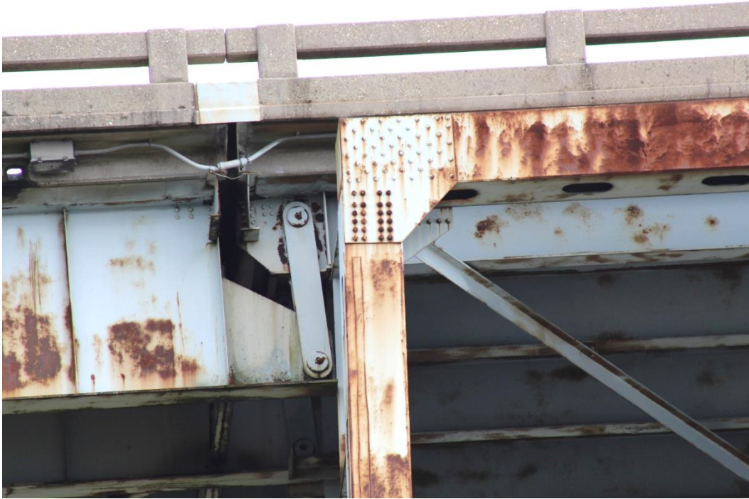
Condition Photo 7: Condition of hinged hangers of plate girders at connection to truss span, with deck expansion joint above the hinge.
