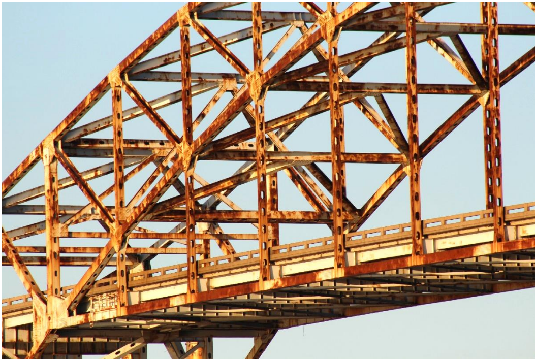
Historic Fabric Photo 4: Portion of suspended truss span, showing floor system components.
