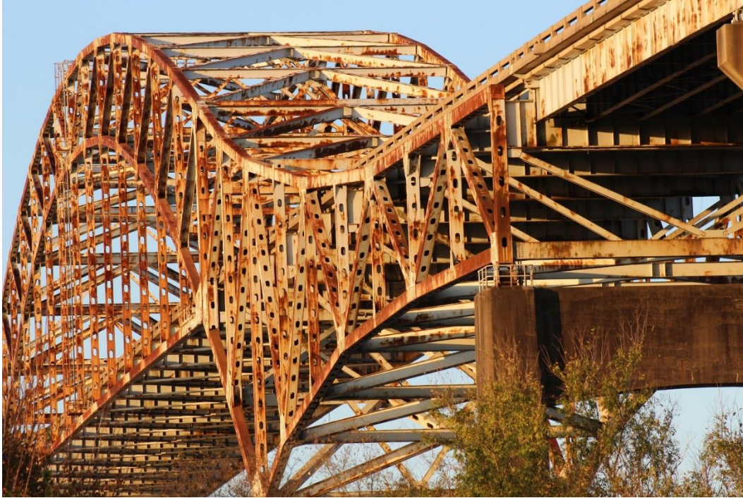
Condition Photo 1: Truss span paint failure.
