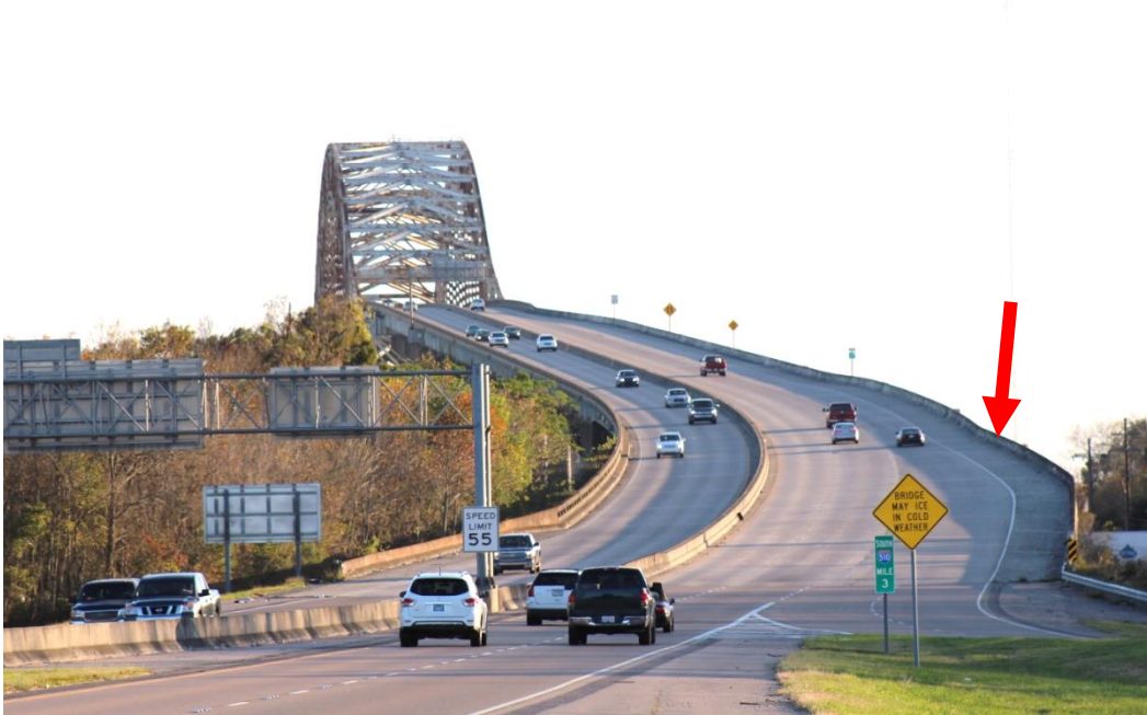
Condition Photo 11: North approach roadway to the bridge, facing southbound direction. Note the on-ramp from Old Gentilly Road Interchange. Note Jersey-style concrete parapet on right side of road.
